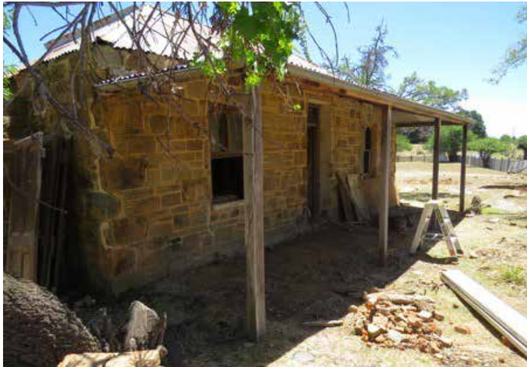
View to NW across front of Denman's Cottage shows where the partially retained brick veranda floor was removed. (Gina Scheer 13.11.2019)
