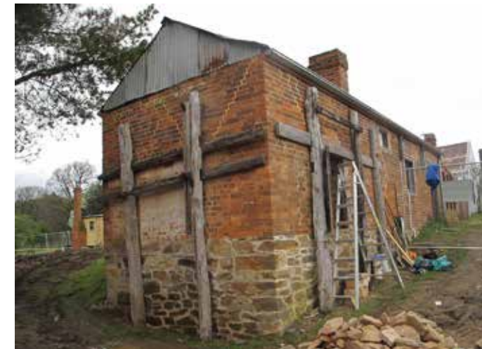
The old bakery (c.1890s) behind the General Store in Hill End (Gina Scheer, 14.09.2016)
