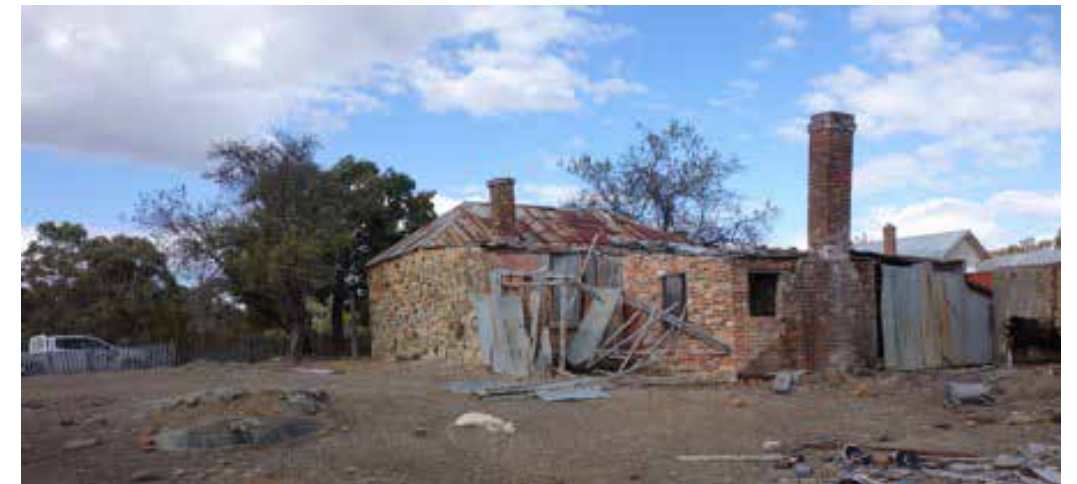
View to SE of the rear and N side of Denmans Cottage prior to the 2019 works. (Gina Scheer,
