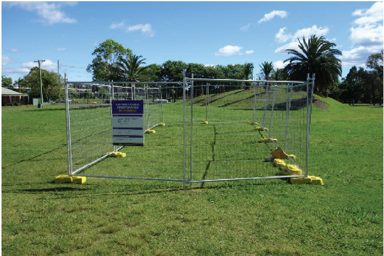
Looking north in the northern section of the LPMP, Hume Highway at background behind the LCC created mound with palm trees. One of the five areas to be excavated in foreground.
