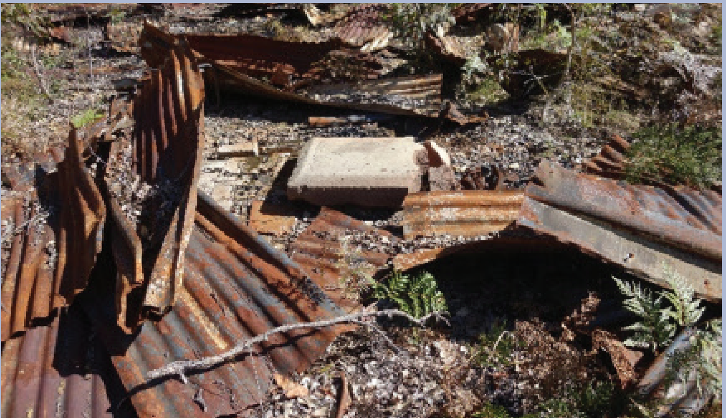
Sandstone step of Pine Creek Hut located amongst debris after fire destruction.
