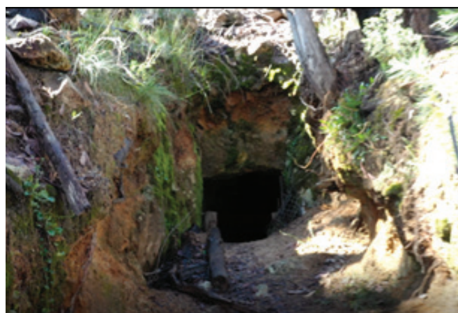
Figure 4: View from the 2022 Assessment of entrance to tunnel, with no wooden elements in place.
